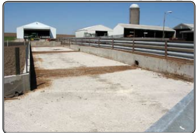
Runoff from the feedlot, at right, travels across the sloped collection ramp and into the sediment basin, at left. The ramp was built wide so that the farmer could drive his tractor through it.
