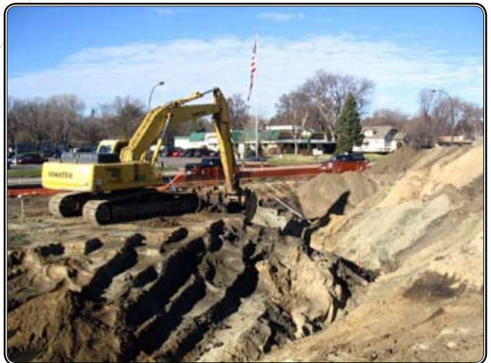
Contaminated soil excavation was required for some of the land on the 13-acre Lyndale Green site.
