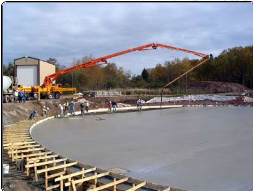
Environmental cleanup was required where this new Two Harbors equalization tank was constructed.
