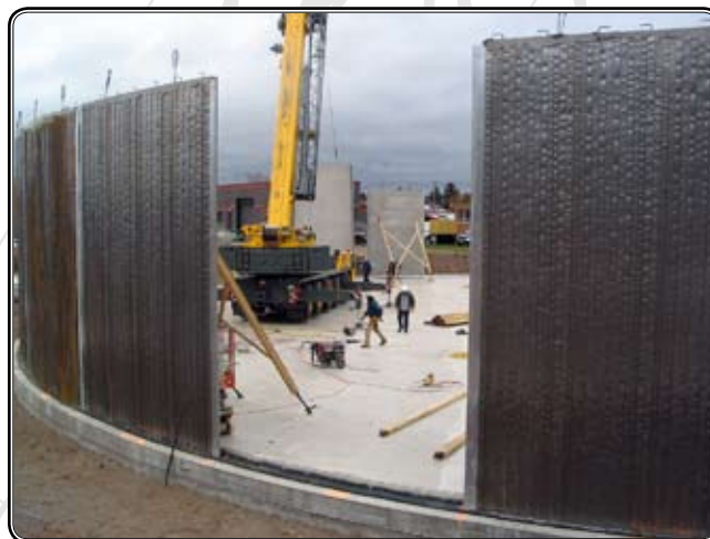
A concrete equalization tank in Two Harbors, MN stores influent from sanitary sewer overflows, preventing untreated water from flowing into Lake Superior. (See related article on Page 6.)
